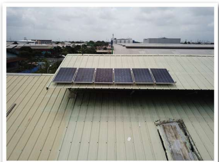
@ Daanmogot - 1 kW On Grid
