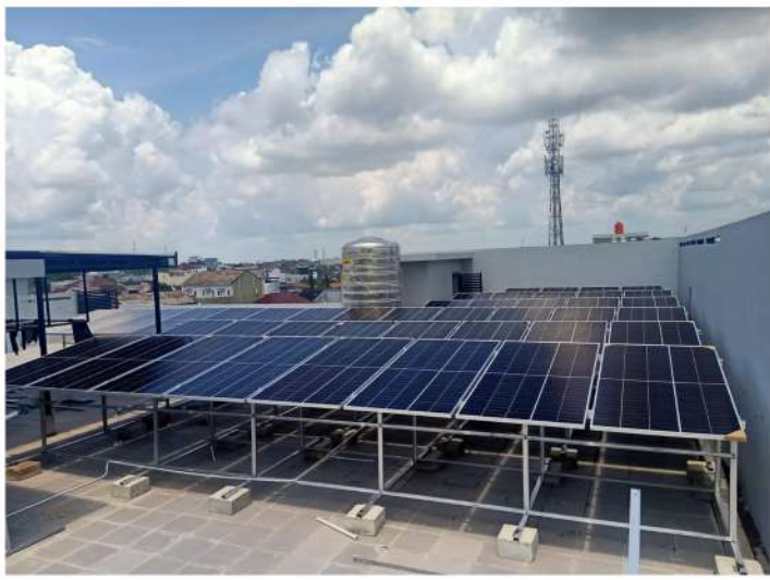
@ Palembang - 30 kW On Grid
