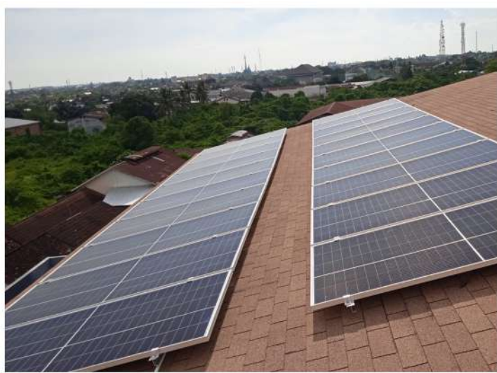
@ Lombok - 10 kW On Grid
