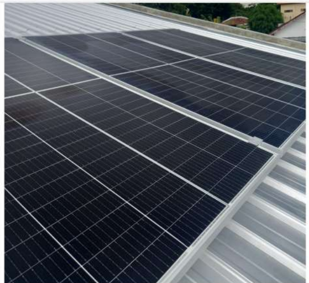
@ Klaten - 5 kW On Grid
