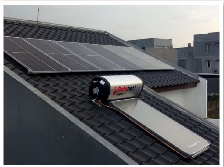
@ Bintaro - 3 kW On Grid
